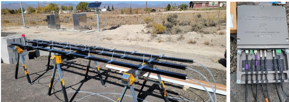
Figure 2 – VectorSense Sensors and Electronics for TACS Installation, Osino, NV
