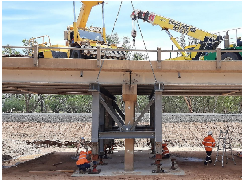
Figure 5 Alice River bridge: Fitting jacking frames to rectify 120mm of pier settlement. (Source: Copyright of the Department of Transport and Main Roads, Queensland, Australia)
