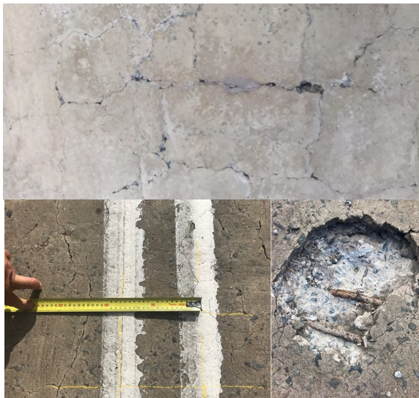
Figure 6 Bee Creek bridge deck slab deterioration
