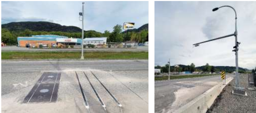
Figure 3 – SLC WIM Scales and VectorSense Sensors at Terrace, BC Virtual Weigh Station
